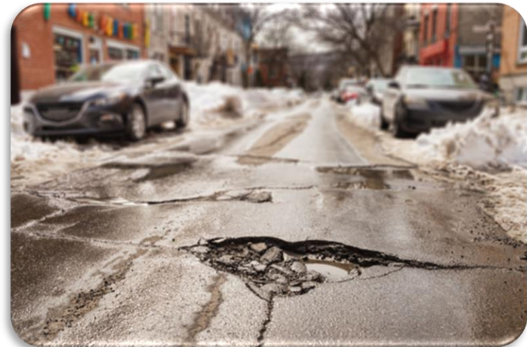
A road crack.
